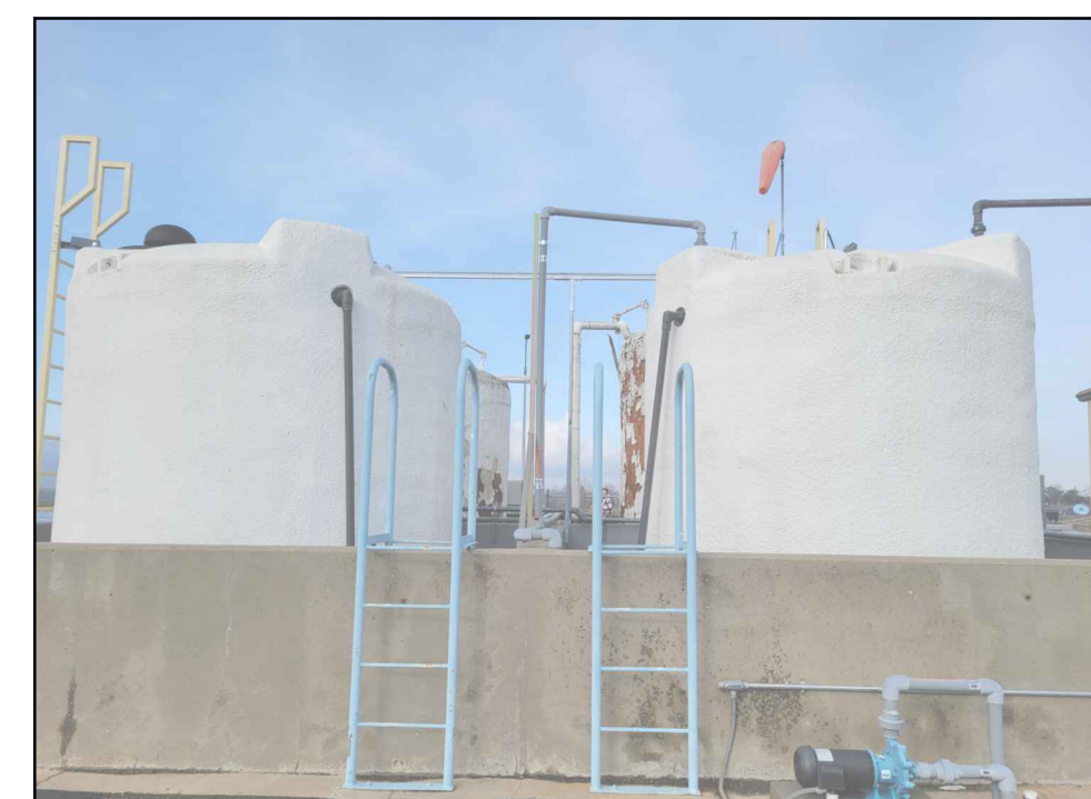
IMAGE NO. 5 SODIUM HYPOCHLORITE STORAGE TANKS
