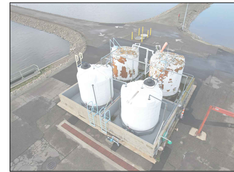
IMAGE NO. 1 AERIAL VIEW OF STORAGE TANKS
