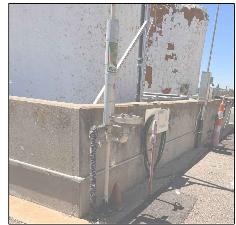
IMAGE NO. 3 EMERGENCY EYEWASH STATION / HOSE RACK
