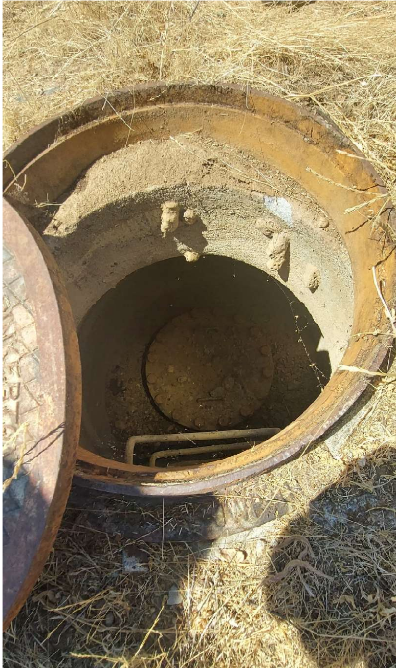
Figure 6-4: Access Hatch to 33" Raw Water Transmission Main
